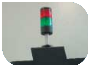
Process control lamp
